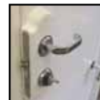
Lockset on watertight door
